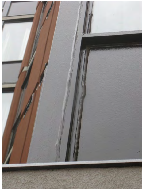
Photo 1: Example of workmanship variations in cap-sealed metal joints.
