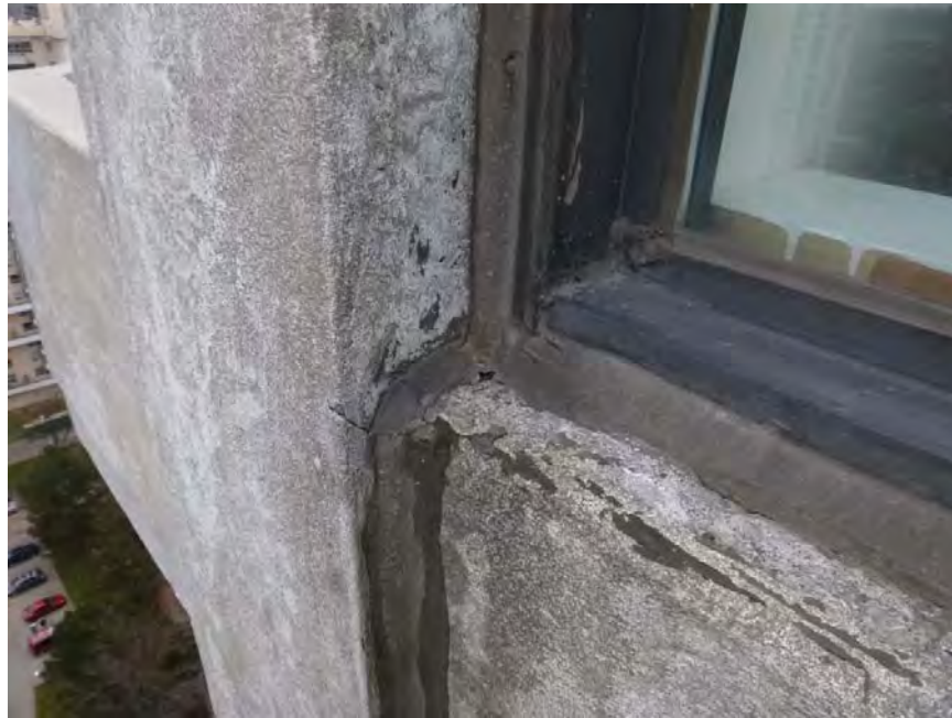
Photo 21: An example of a localized section of debonded window perimeter sealant.
