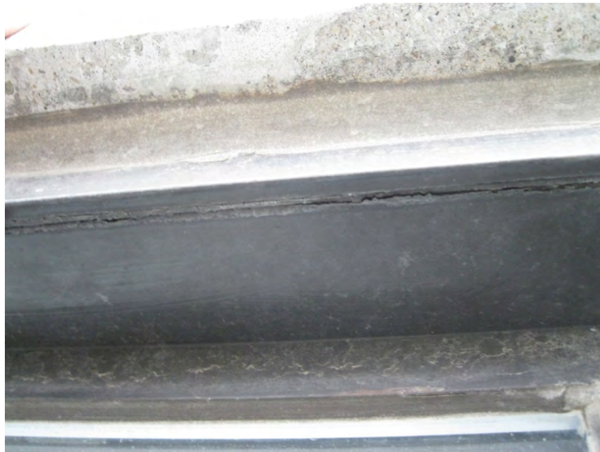
Photo 24: Another example of failed metal-to-metal sealant at a window head.
