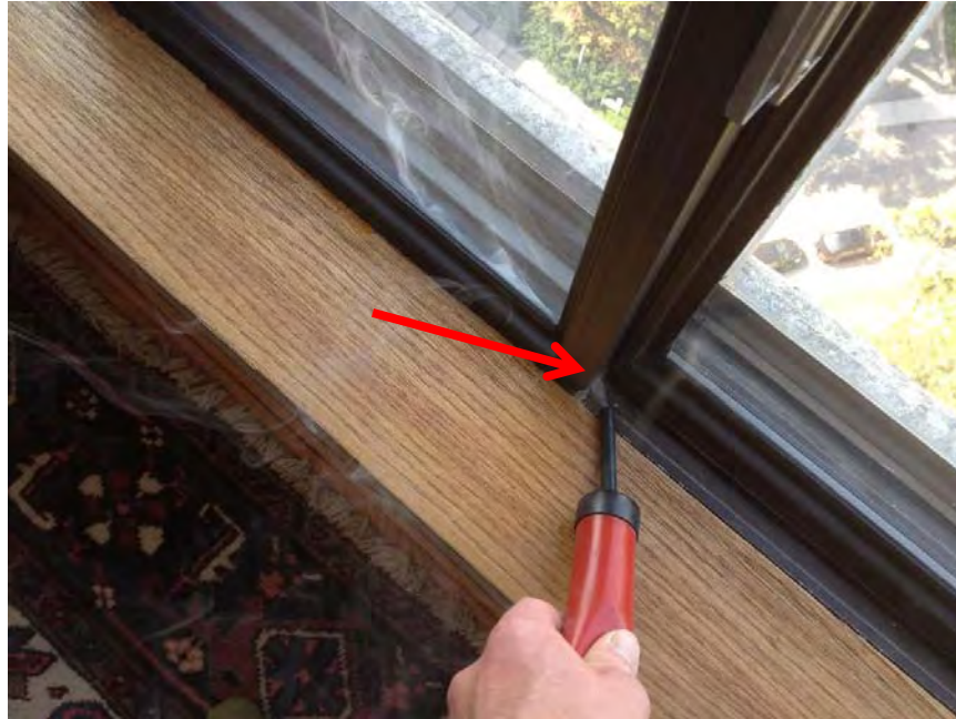
Photo 13: Using a smoke pencil, we noted widespread air leakage at operable windows – note the smoke travelling through the closed operable window at the bottom of the meeting style (red arrow).
