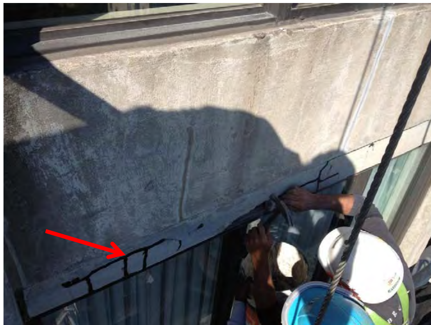
Photo 10: Photo of concrete repair work under way. Concrete fractures have been previously sealed over using brown sealant (red arrow). Brook is completing a repair at a previously sealed location.
