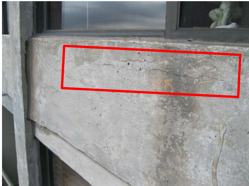
Photo 8: An example of a fractured and delaminated concrete (red box) at a concrete cladding panel below a window.
