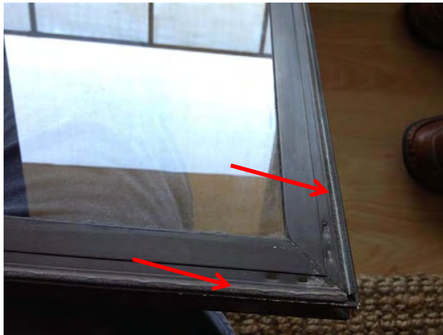
Photo 14: Fin type weather stripping at operable windows appeared to be in generally serviceable condition.
