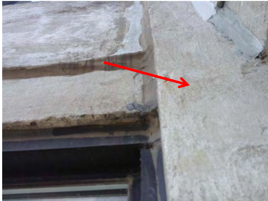
Photo 11: An example of a wall to floor slab construction joint is identified with a red arrow.
