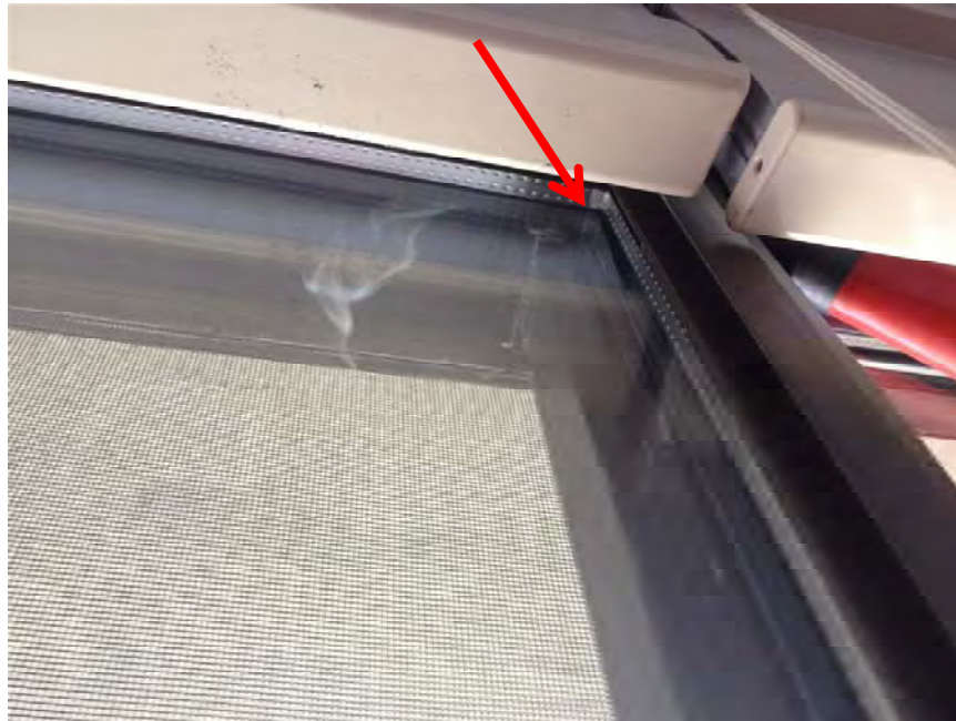
Photo 17: Air leakage was also noted at the top and bottom corners of sliding doors. Note the smoke travelling through the top corner of a closed sliding door (red arrow).
