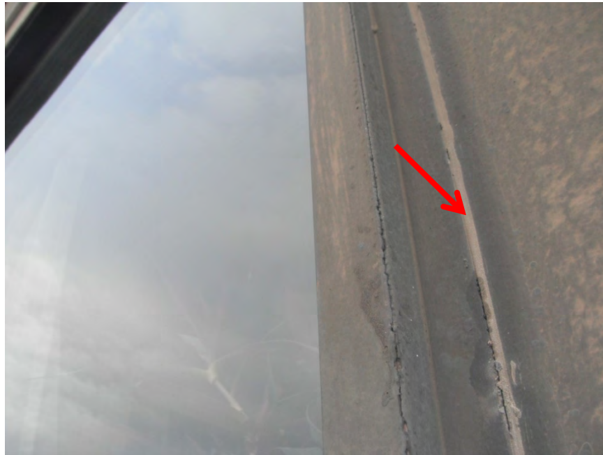
Photo 25: The profile of the needle glazing at metal cladding panels (indicated with red arrow) is generally thin and narrow.
