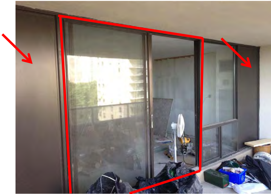
Photo 3: An example of a window wall assembly at a recessed balcony location. The sliding balcony door that is inset into the window wall frame is identified with a red box. Metal cladding panels are identified with red arrows.
