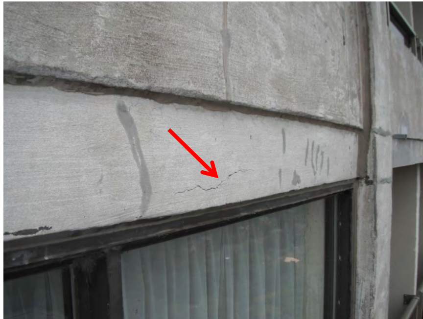
Photo 7: An example of a fractured concrete floor slab above a window location (red arrow).
