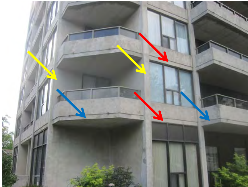
Photo 5: Structural concrete floor slabs (red arrows), balcony slabs (blue arrows), and shear walls (yellow arrows) are exposed at typical locations.
