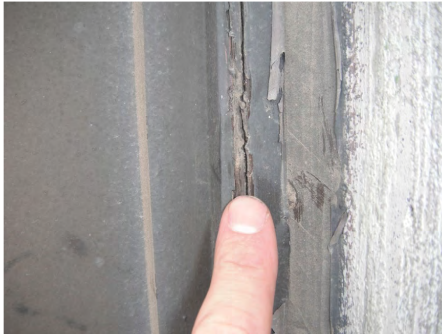
Photo 23: An example of failed metal-to-metal sealant at a window jamb.
