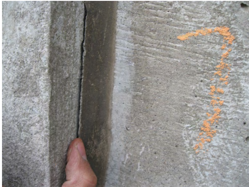
Photo 22: An example of a debonded sealant joint at a precast panel perimeter.
