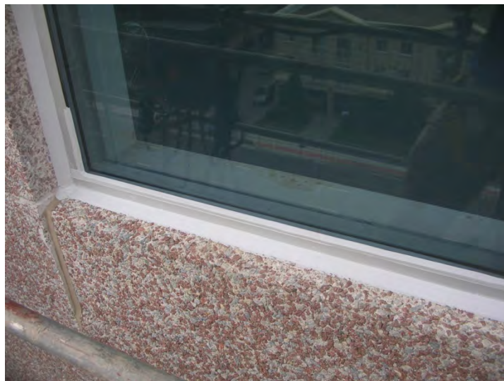
Photo 2: Example of cap seal at glass/metal joint limited to bottom of IGU.
