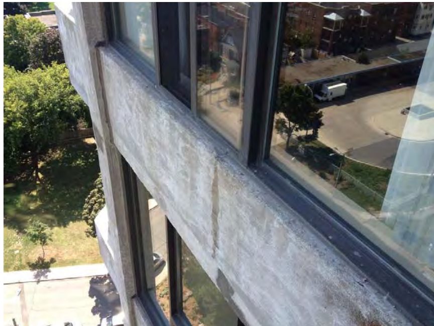
Photo 12: Operable window drainage performance was variable throughout the building. In this location, only 1 of 4 drains was functioning, as confirmed by pouring water into the window track.
