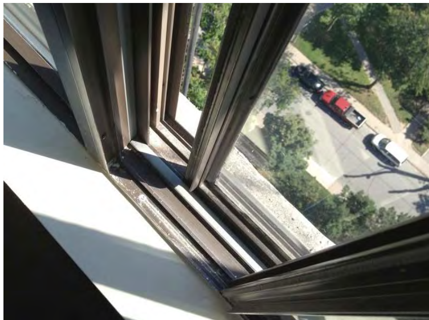
Photo 16: An example of a worn window track; likely a result of worn out rollers.
