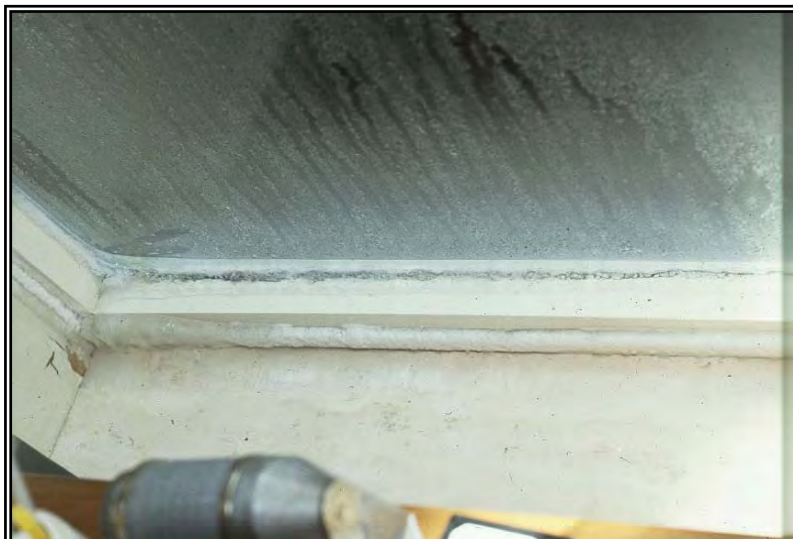
Photo 1.: Example of severe condensation from thermal bridging, excessive humidity and poor heat distribution.
