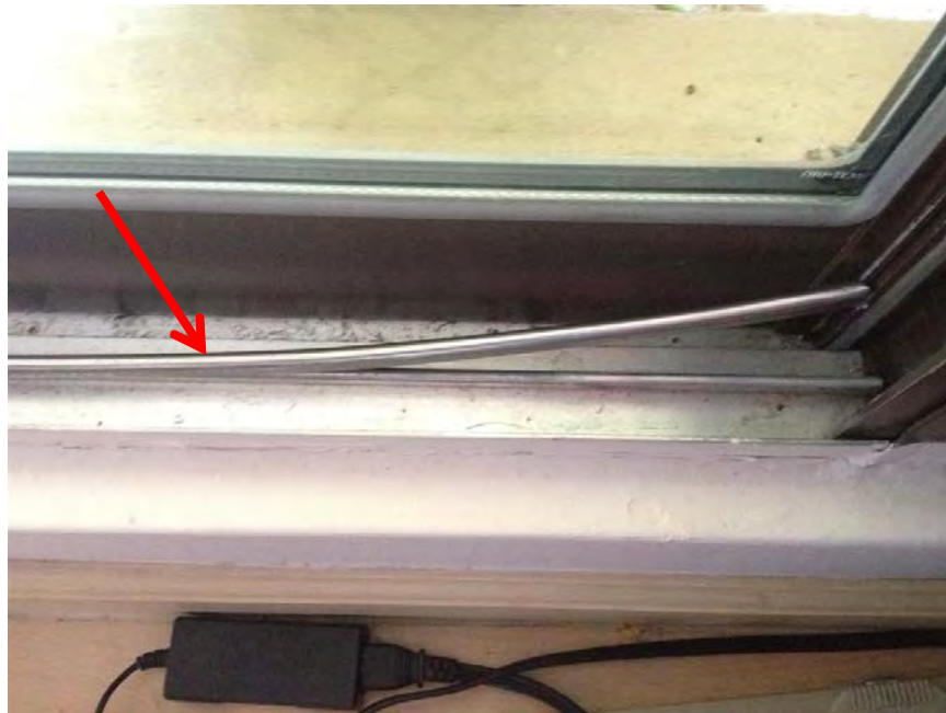
Photo 20: New stainless steel sleeves (red arrow) have been installed at some sliding door locations. In some places, the sleeve has become bent and is no longer functioning as intended, as shown in the photo above.
