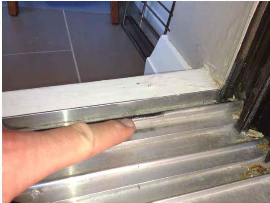
Photo 19: An example of a sliding door track that is severely worn.
