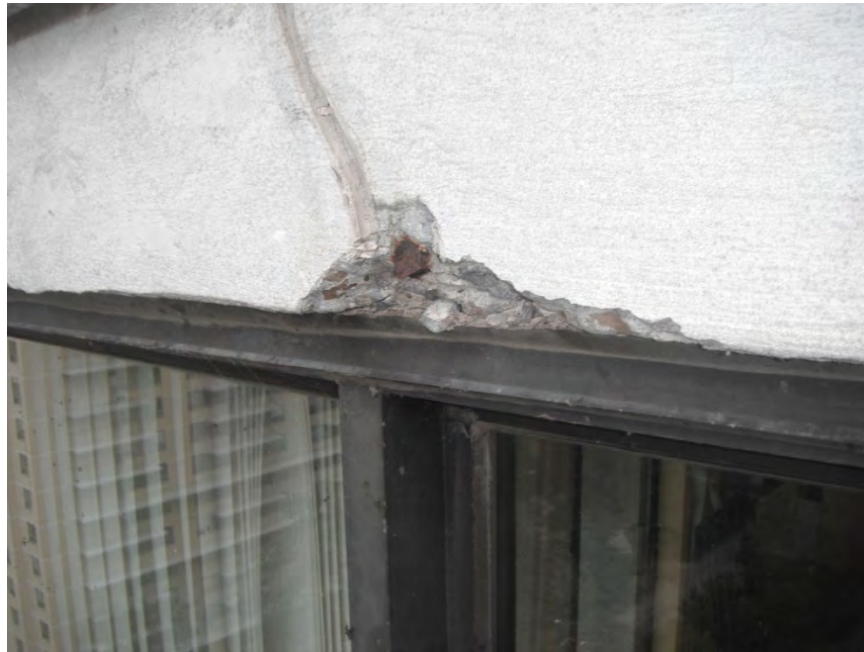
Photo 9: An example of a concrete spall due to corrosion of reinforcing steel in exposed concrete floor slabs.
