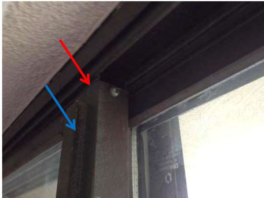
Photo 18: The existing door perimeter and meeting style weather stripping (blue arrow) is in generally poor condition and no dust plugs were present at door corners (red arrow indicates where dust plug should be).
