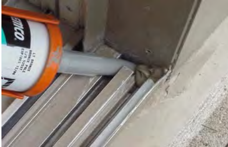
Photo 3: Example of challenging retrofit seal at operable sill corner
